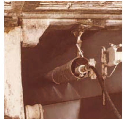
Electrically driven traverse beam with fan nozzles
